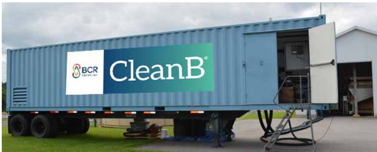
Figure 1: CleanB® Demo Unit installed at Mebane Bridge WWTP
